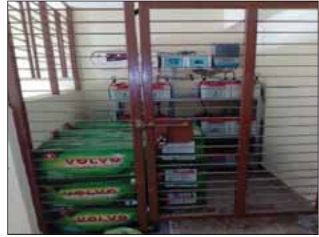
Emergency Power Supply of Multipurpose Disaster Shelter (Bhola Sadar)
