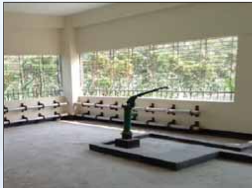
Drinking Water Facility of Multipurpose Disaster Shelter (Bhola Sadar)
