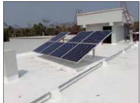
Emergency Solar Power Supply of Multipurpose Disaster Shelter (Gournadi Barishal)
