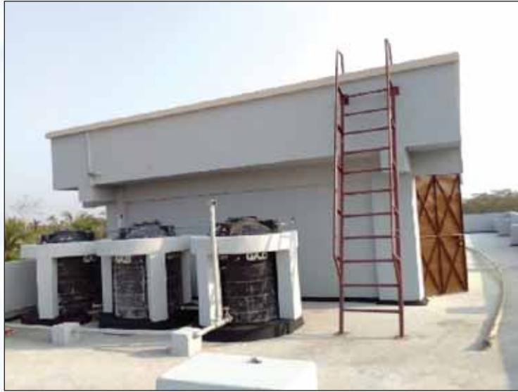
Water Preservation Tank of Multipurpose Disaster Shelter (Borhanuddin, Bhola)
