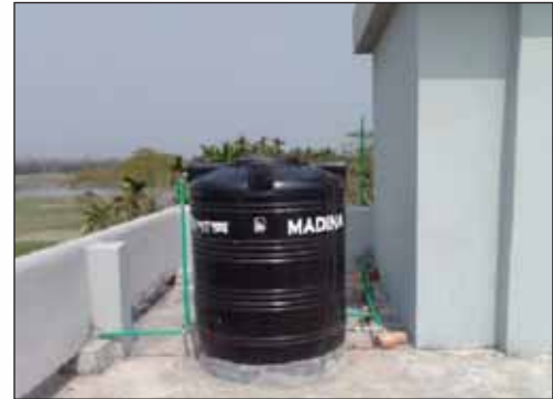
Water Preservation Tank of Existing Multipurpose Disaster Shelter (Daulatkhan, Bhola)
