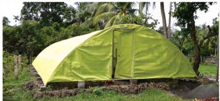
Net Shed Constructed at Barguna Horticulture Centre under ASSSRBP with the supervision of Design & Supervision Consultant
