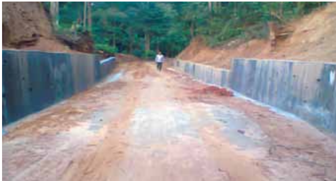
△ CDMP intervention near Union Parishad Bhaban at Baishari village of Naikhyongchari Upazila in Bandarban district
