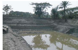
Shopon Chokidar's home pond excavation in Royanda union, Sarankhola Upazila of Bagerhat.
