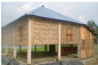
Construction of flood resilient house and plinth raising in Uttur Durung union, Moeshkhali Upazila of Cox's Bazar district.
